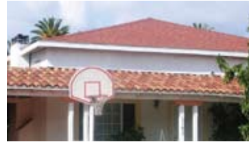
Part of the original clay tile roof has been changed to asphalt shingle.
