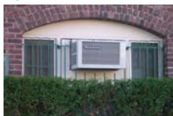
The original arched opening has been filled in with an air conditioner and smaller windows.
