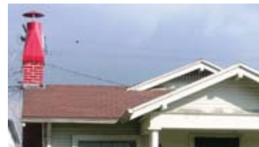
The altered chimney detracts from this charming Craftsman home.
