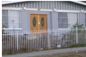
The original Craftsman porch was inappropriately filled in.
