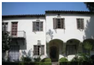
These wood casement windows have thin, delicate grids and are recessed in the openings.
