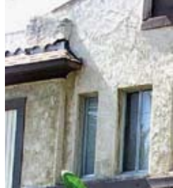
The heavily textured stucco attracts dirt.
